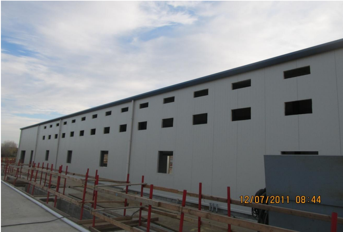
Balfour Beatty subcontractor Quality Erectors cutting out HVAC openings in the control building.
