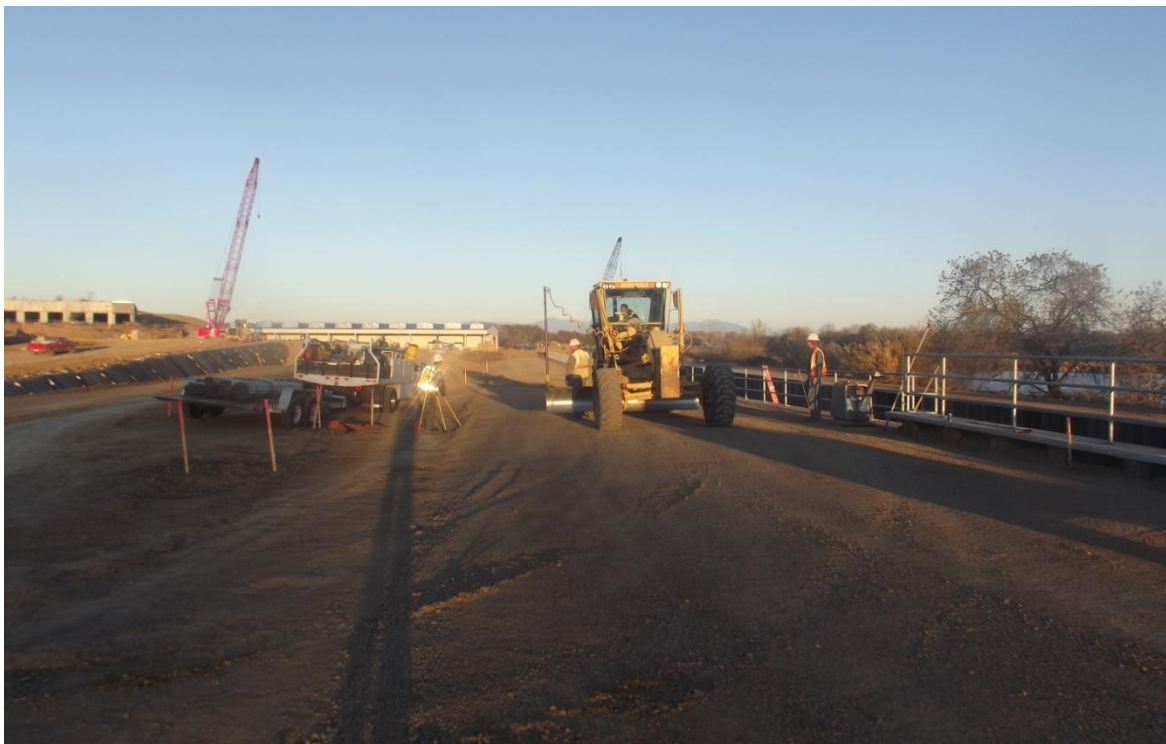
West Bay Builders subcontractor Meyers grading the gravel surfacing of the A1 Line Road.
