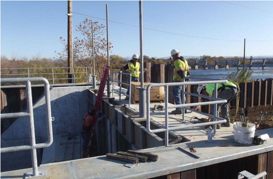
West Bay Builders subcontractor Blue Iron finishing installation of handrail at the Inlet Structure.
