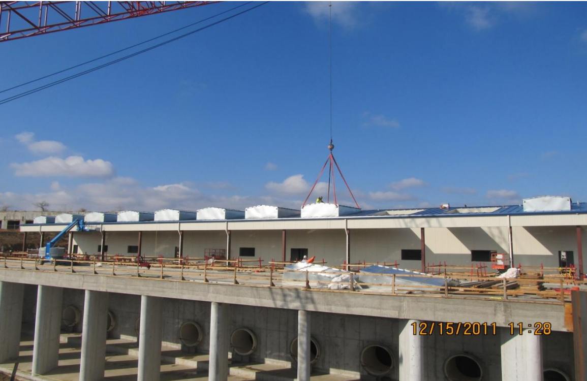
Balfour Beatty subcontractor Quality Erectors setting and installing roof hatches on the control building.
