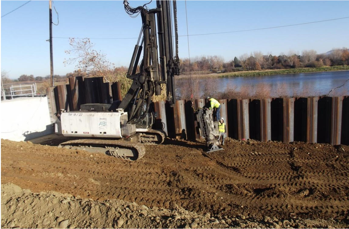
West Bay Builders subcontractor Blue Iron preparing ABI machine to remove temporary sheet pile.
